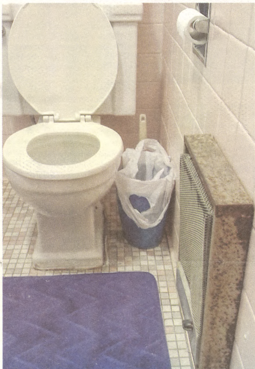
The focus of the renovations to Georgia Hall will be on the outdated and rusty bathrooms.
